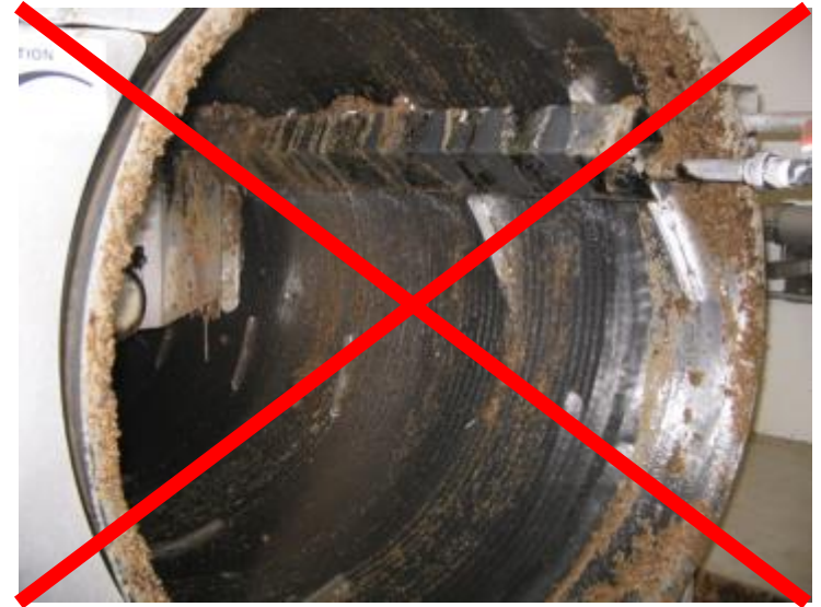
No Screening Prior to Treatment System
