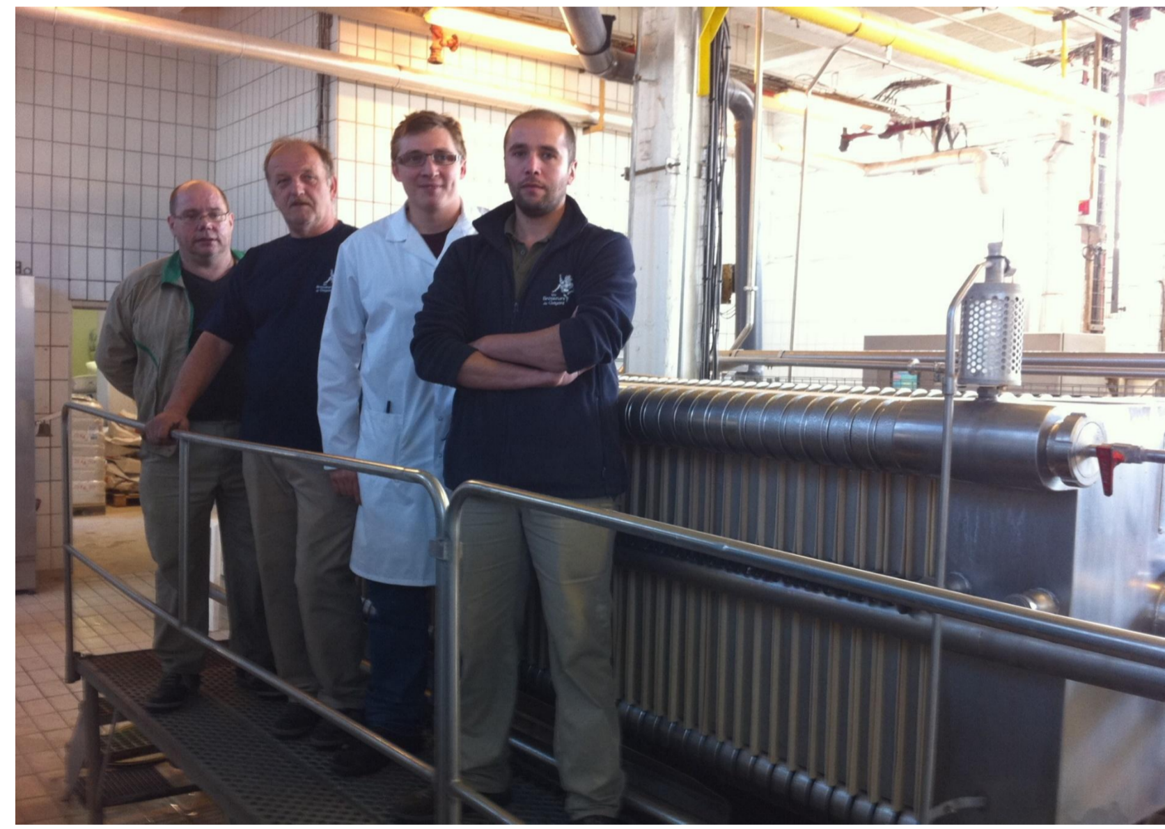
68m 2 frame filter with DE free single pre-coat and bodyfeed.
